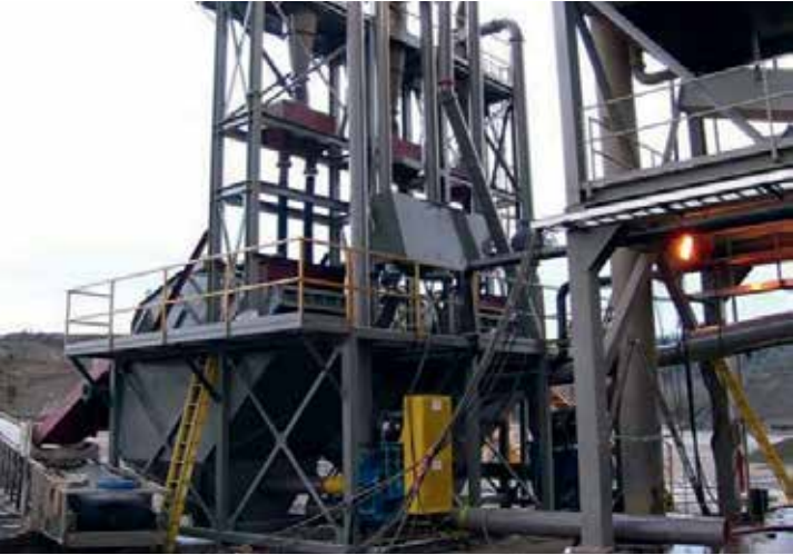
Hydrocyclone tower – HR
