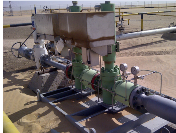
Mechanical HIPPS skid in Saudi Arabia.
